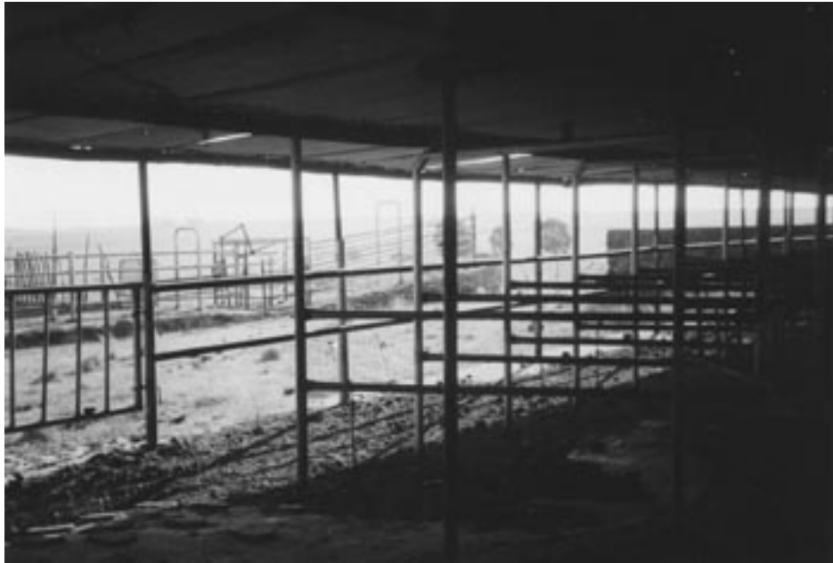
The broken dairy pens at a non-functional dairy – the farm Leeupoortjie, Botshabelo, after the handover.
